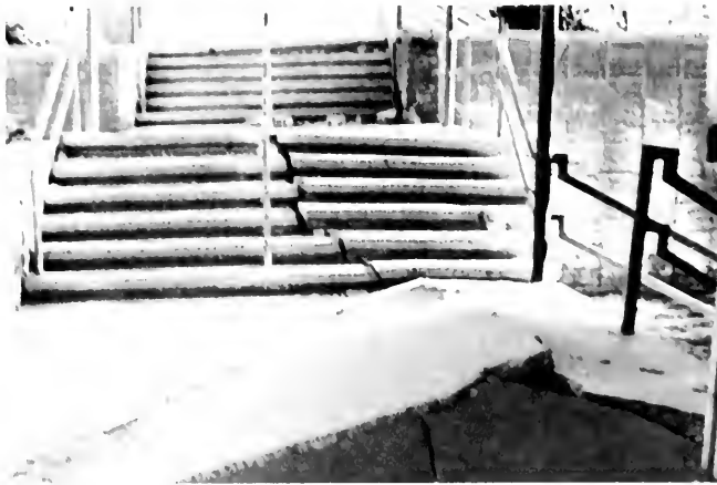
Photo 16. Sylmar High School. The site had considerable ground fissures.
